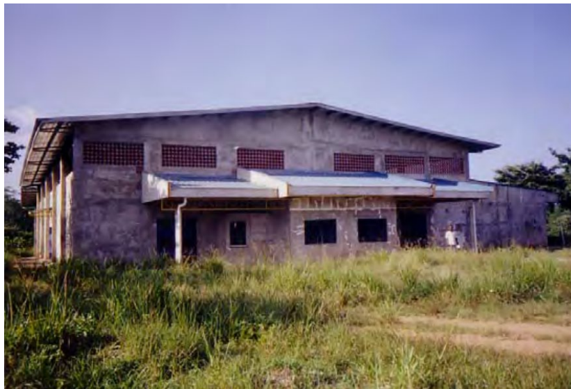
FIGURE 13 A PAST MUNICIPAL GOVERNMENT ADMINISTRATION BUILT BUT DID NOT FINISH THIS GYMNASIUM/MULTIPURPOSE COMPLEX NEAR LA PALMA IN 2001
